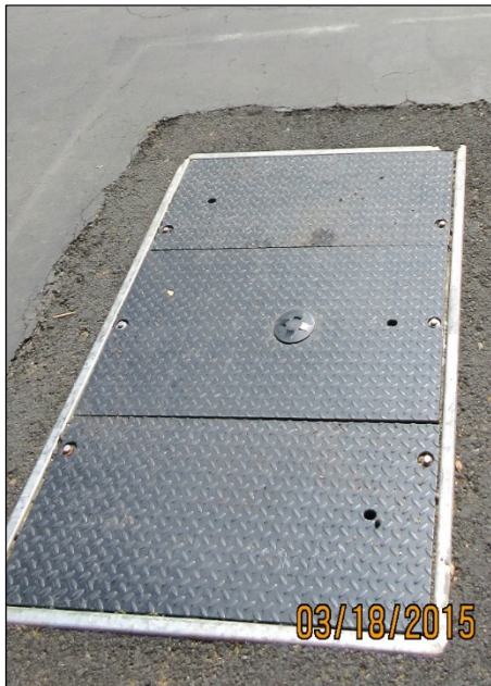
Figure 2 EGWD Typical Meter Boxes with Thru-pit Touch Pad
